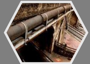
OVER 20,000 MILES OF PIPES Water & wastewater
