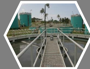
AROUND 3,800 AUXILIARY FACILITIES, INCLUDING: TANKS - 1,564 PUMP STATIONS – 1,966 WATER WELLS - 238
