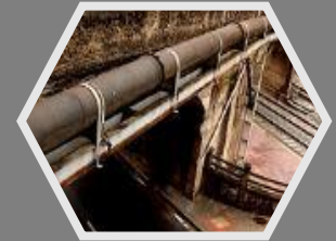
OVER 20,000 MILES OF PIPES
