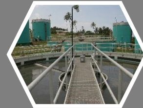
OVER 3,900 AUXILIARY FACILITIES, INCLUDING: TANKS - 1,563 PUMP STATIONS – 1,972 WATER WELLS - 238
