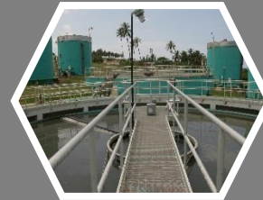
AROUND 3,800 AUXILIARY FACILITIES, INCLUDING: TANKS - 1,568 PUMP STATIONS – 1,966 WATER WELLS - 238
