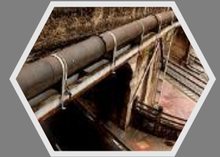
OVER 20,000 MILES OF PIPES Water & wastewater
