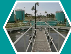
AROUND 3,800 AUXILIARY FACILITIES, INCLUDING: TANKS - 1,569 PUMP STATIONS – 1,966 WATER WELLS - 244
