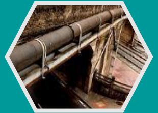
OVER 20,000 MILES OF PIPES Water & wastewater
