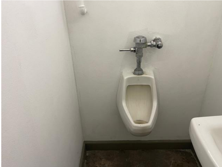
Bathroom 1- Ceramic Urinal with Lead Based Paint
