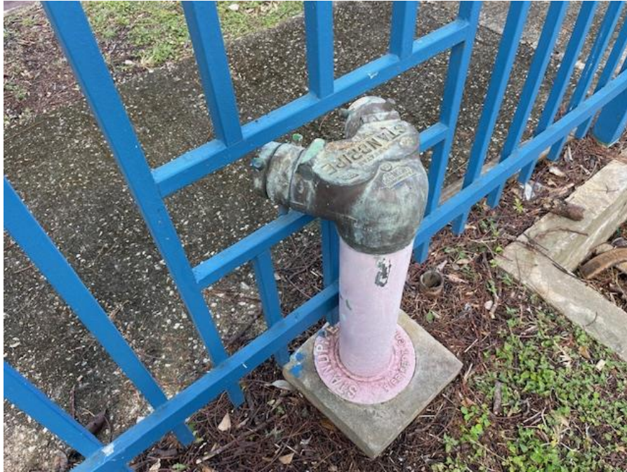
Exterior- Side D- Metal Fire Hose Connection with Lead Based Paint
