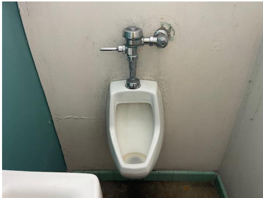
Bathroom 4- Ceramic Urinal with Lead Based Paint
