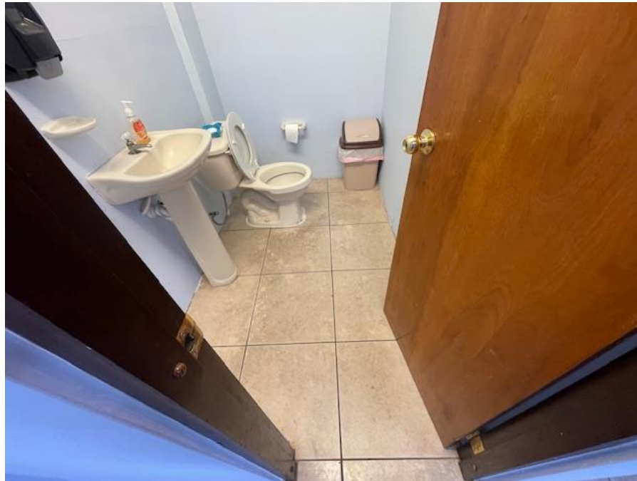
Bathroom 2- Ceramic Floor Tiles with Lead Based Paint
