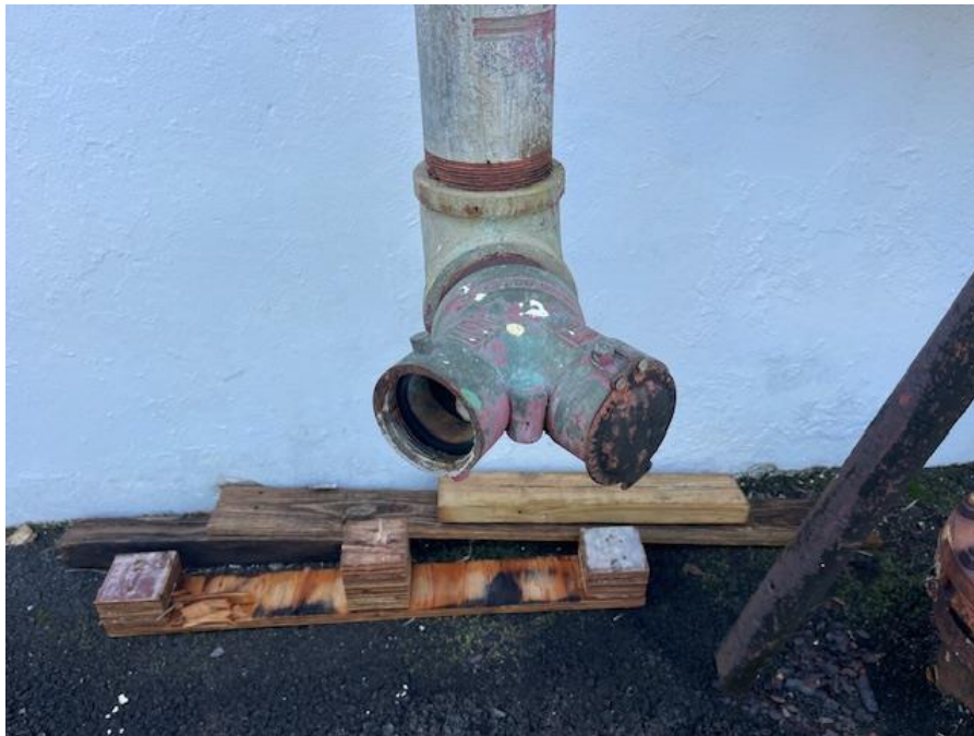
Exterior- Side B- Metal Fire Hose Connection with Lead Based Paint
