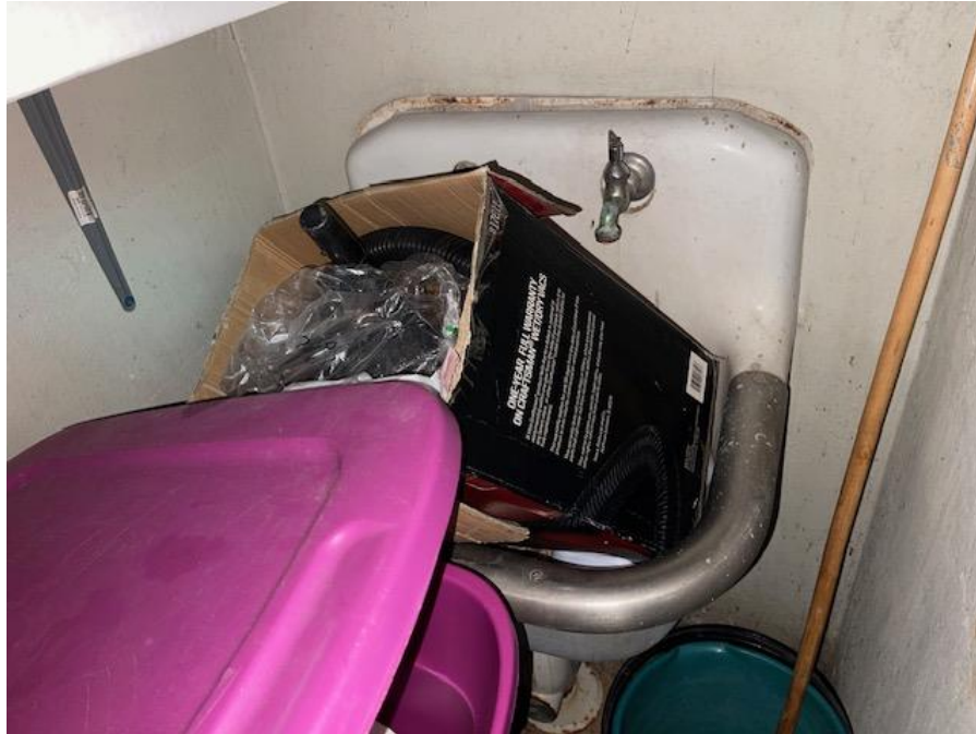
Janitor 2- Ceramic Sink with Lead Based Paint
