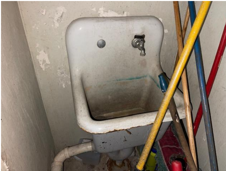
Janitor- Ceramic Sink with Lead Based Paint
