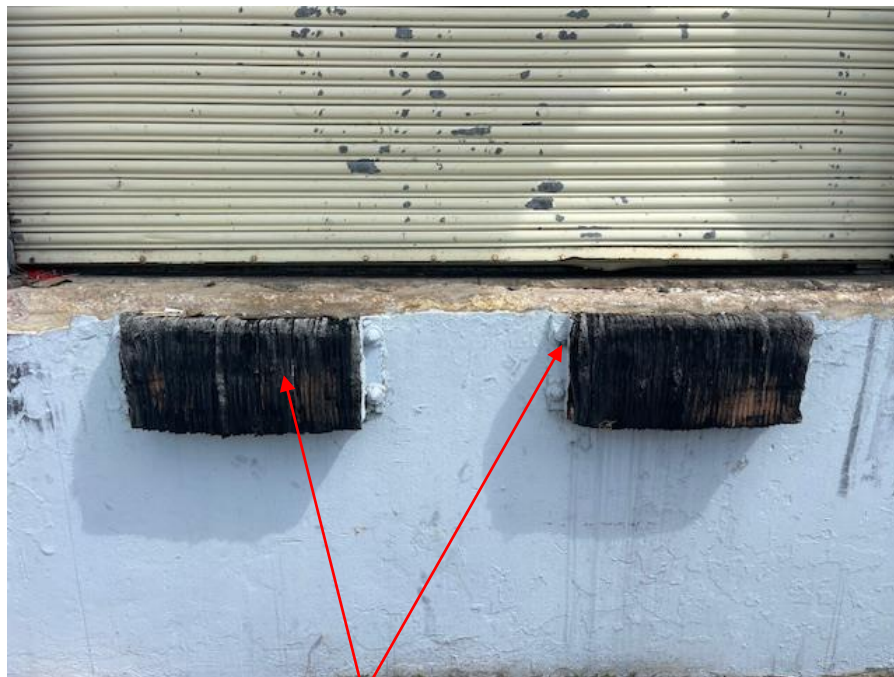
Exterior-Side D- Metal Barrier Plates with Lead Based Paint
