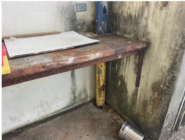
Loading Dock- Yellow Area (5) Five Metal Columns with Lead Based Paint
