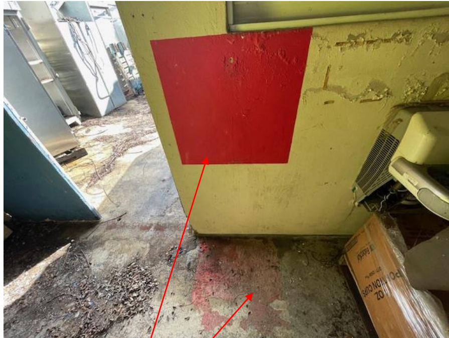
Room 41- Red Concrete Wall & Floor Extincter Area with Lead Based Paint
