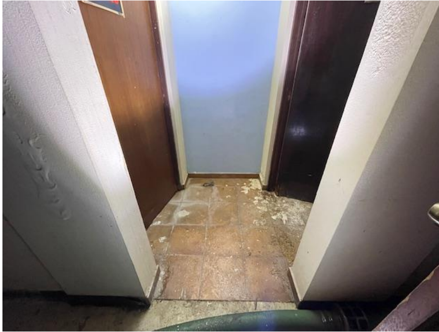
Hallway 5- Ceramic Floor Tiles & Baseboards Tiles with Lead Based Paint
