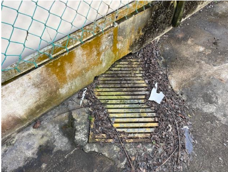
Room 40- Metal Grill with Lead Based Paint
