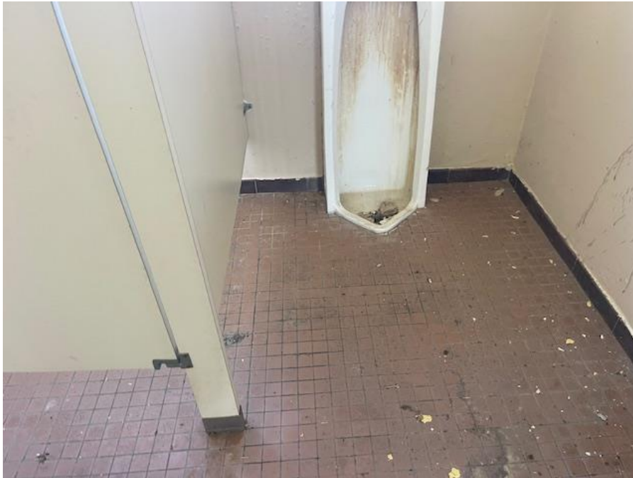
Bathroom 3- Ceramic Baseboards Tiles with Lead Based Paint
