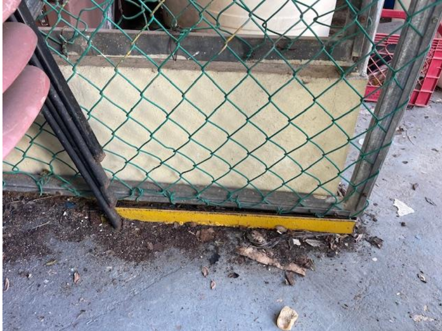
Exterior Room 40- Yellow Metal Base with Lead Based Paint
