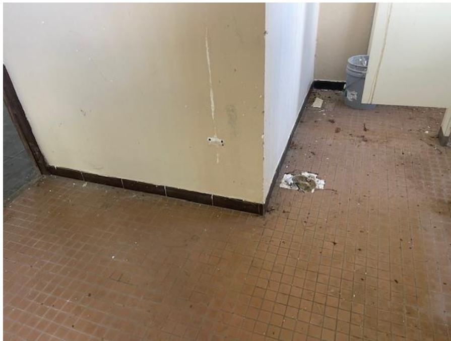
Bathroom 2- Ceramic Baseboards Tiles with Lead Based Paint
