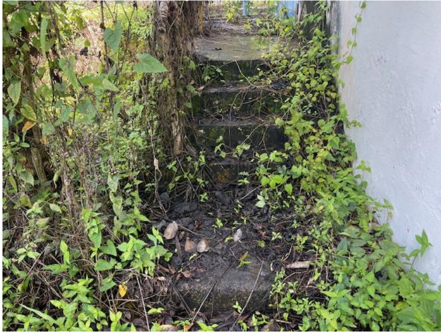
Exterior- Stair- Concrete Floor with Lead Based Paint
