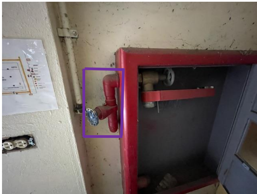
Room 1- Red Metal Pipe with Lead Based Paint
