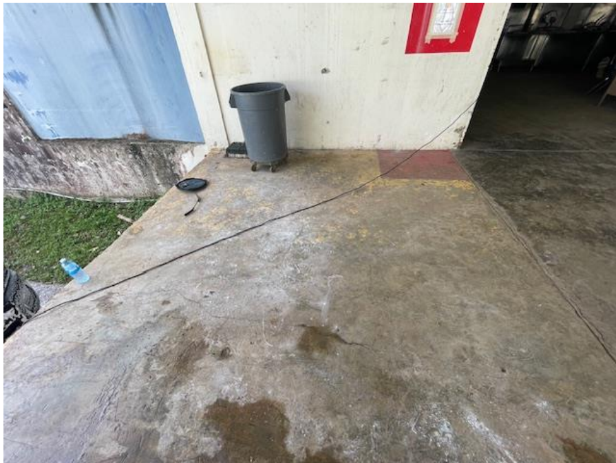
Loading Dock- Concrete Floor with Lead Based Paint
