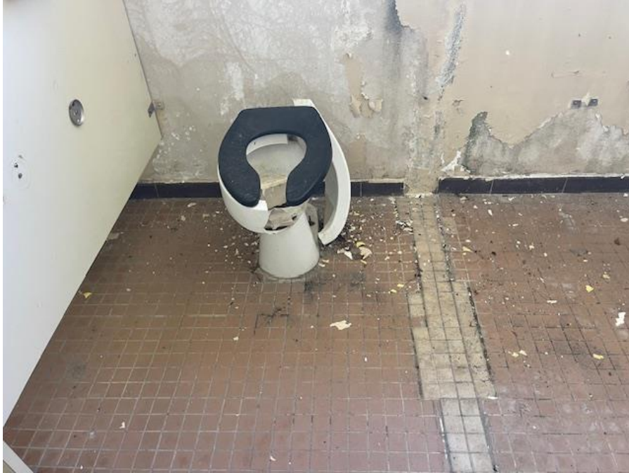
Bathroom 4- Ceramic Baseboards Tiles with Lead Based Paint
