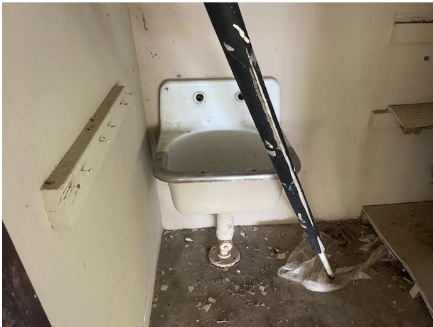
Janitor Room 2- Ceramic Sink with Lead Based Paint
