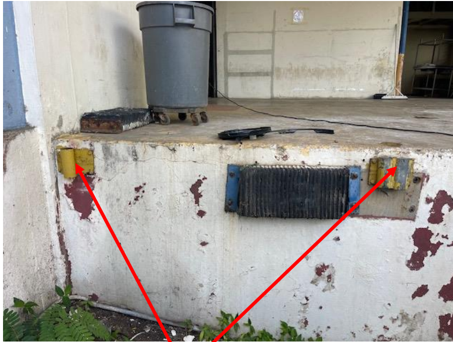
Loading Dock- Yellow Metal Bases with Lead Based Paint
