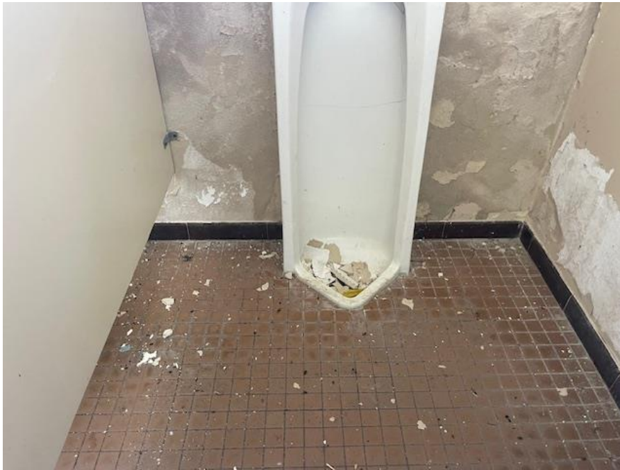
Bathroom 1- Ceramic Baseboards Tiles with Lead Based Paint
