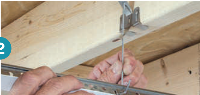
Suspend main beams with hanger wire or QuickHang™ hardware* (shown above: QuickHang hooks and brackets)
