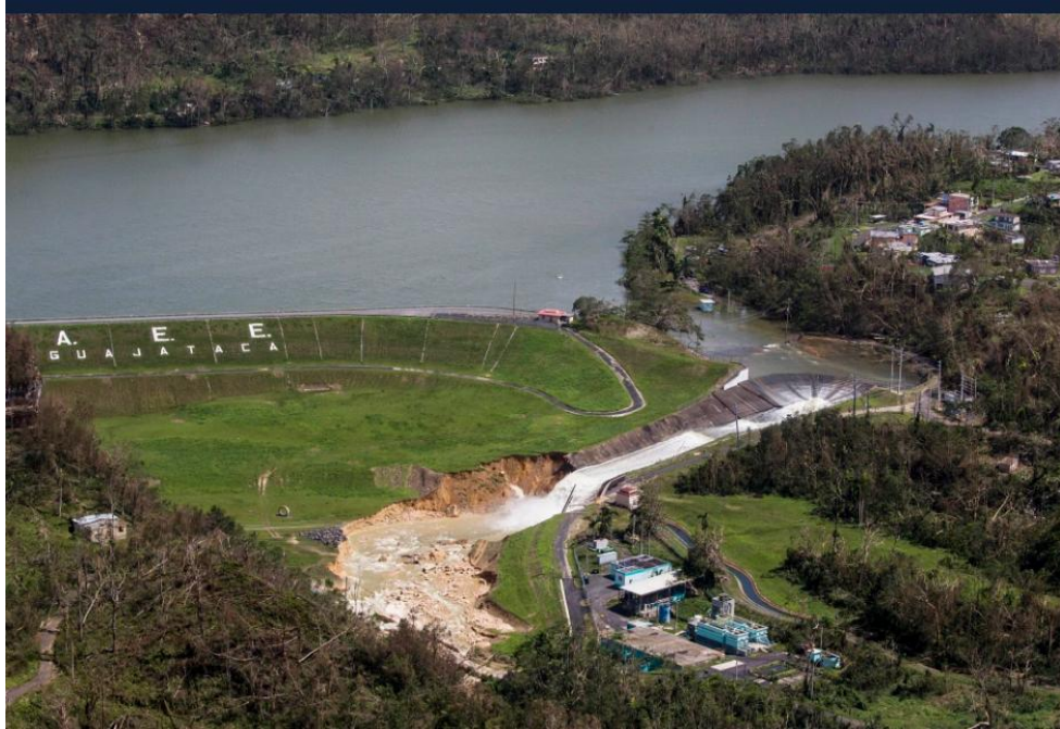
Figure 26: Guajataca Dam Breach 9/23/2017 1
