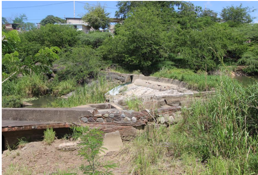
Figure 3. Partial view of a late 1800s dam, water intake and supply canal, built on the Coamo River to provide water for three haciendas: Florida , Santa Isabel and El Destino . (Photographer: Juan Llanes Santos, 2016)
