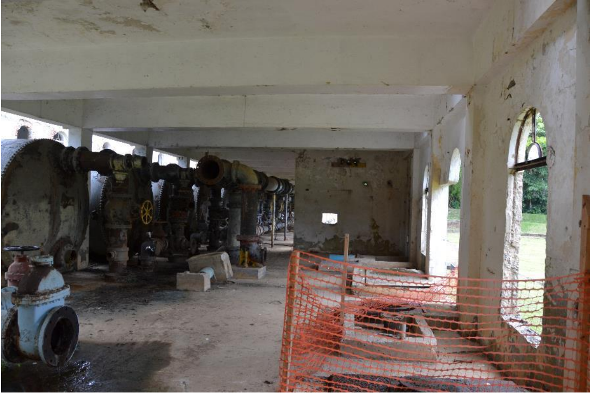
Photo #21: Chemical and Mechanical Filters' House, interior
