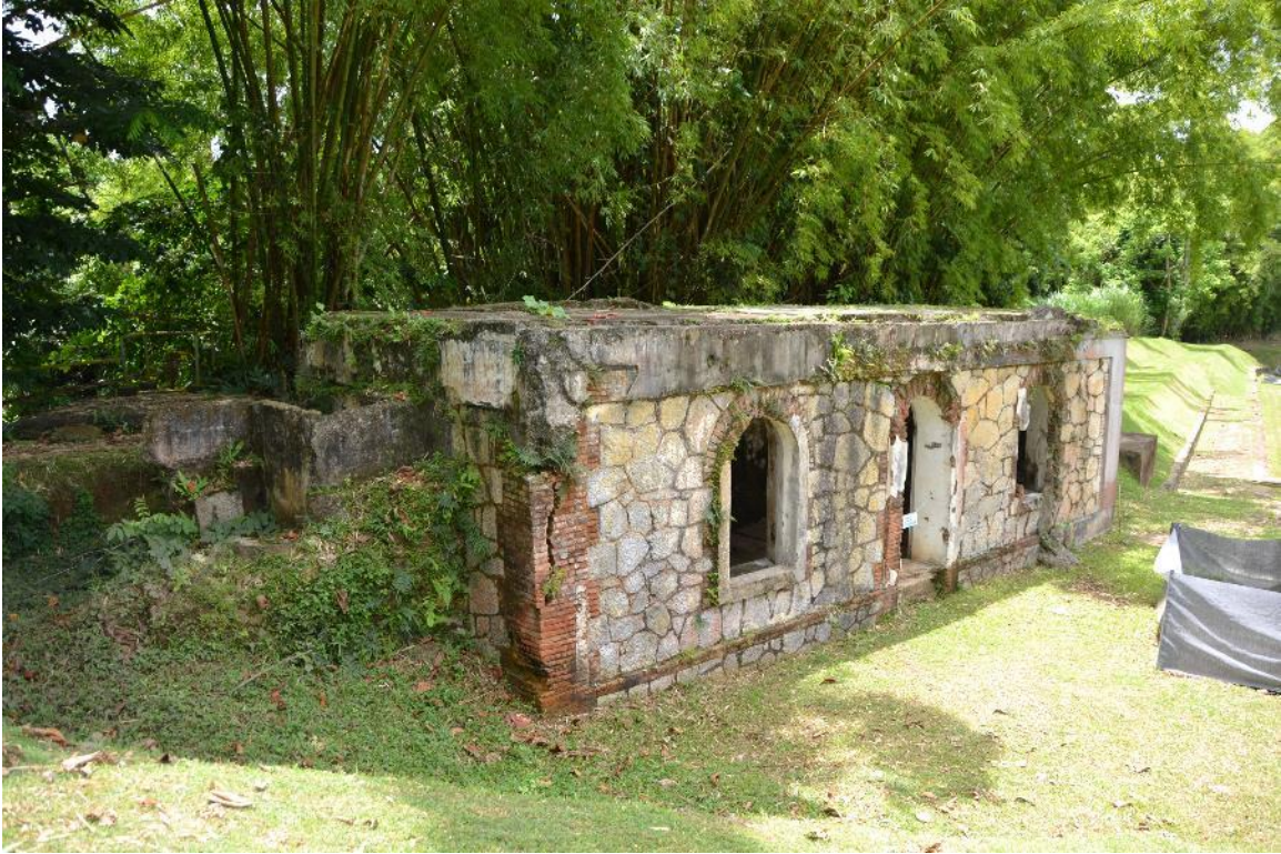
Photo #7: Mixing Chamber and Valve House
