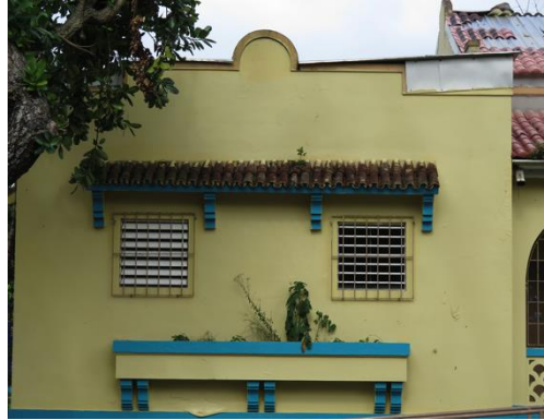
Figure 33. Detail of reinforced concrete cantilevered roof slab eaves, balustrade, plant box and brackets, Building B, 1925-1928, Joseph O'Kelly, Instituto Loaiza Cordero para Niños Ciegos Historic District, APC, 2018.
