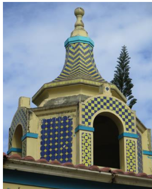
Figure 29. Tower Lantern, Building A, 1925-1928, Joseph O'Kelly, Instituto Loaiza Cordero para Niños Ciegos Historic District, APC, 2018.
