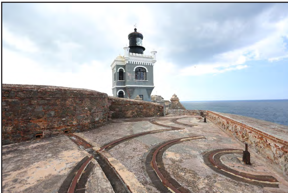
18 Castillo San Felipe del Morro, Ochoa Bastion terreplein and El Morro Lighthouse, looking northwest.
