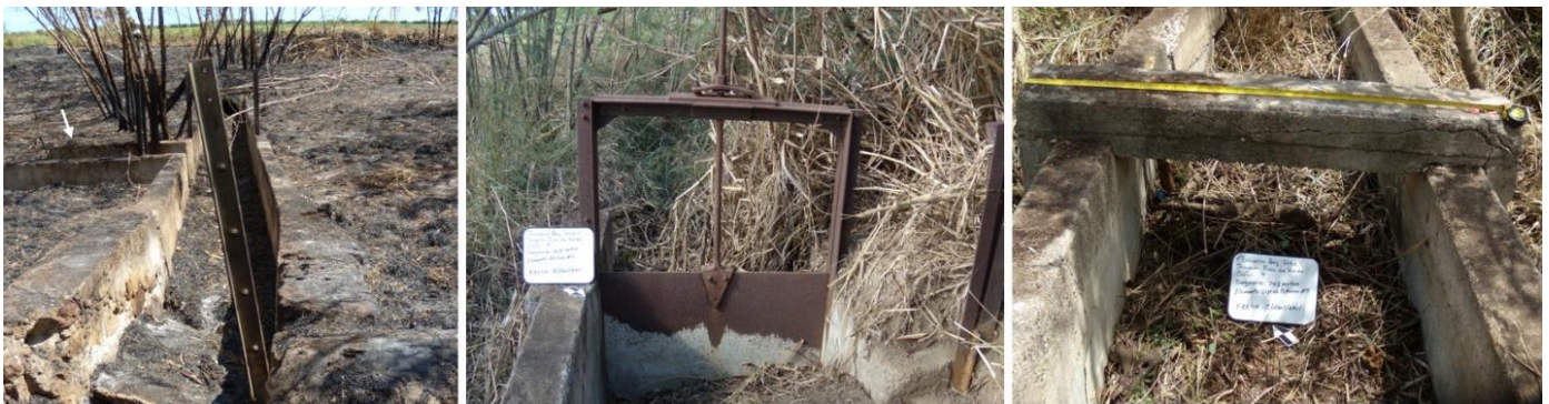
On the left, view of the Hacienda Destino channel, facing west. White arrow shows a channel that was added when it became part of the Irrigation District. In the center, detail of added sluice gate. Right; reinforcement beam added to the Hacienda Florida Channel.
