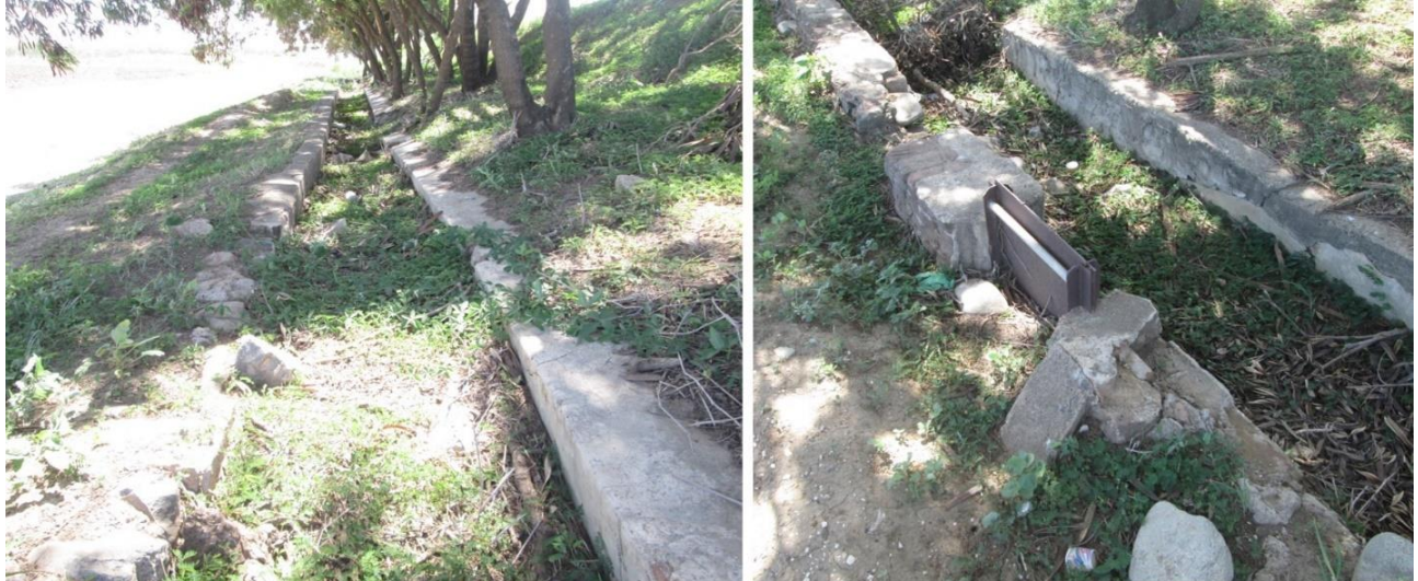
Left; view of the sub-branch, or Channel 5, facing west. Right; detail of the sluice gate.
