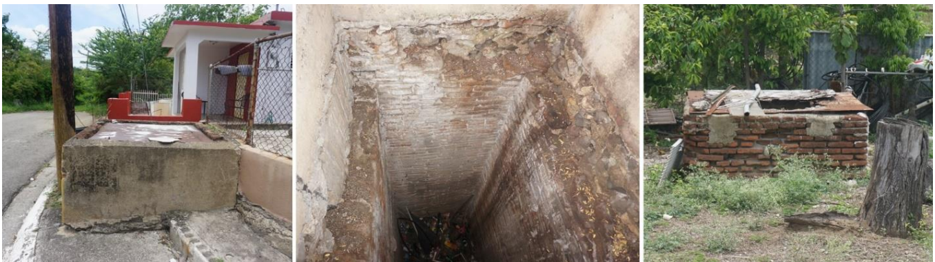
On the left, service manhole to the supply channel, located on a sidewalk of the El Ojo Community. In the center, detail of the service shaft inside a manhole. Right, manhole which features an advanced degree of damage by erosion, located in the backyard of a house.
