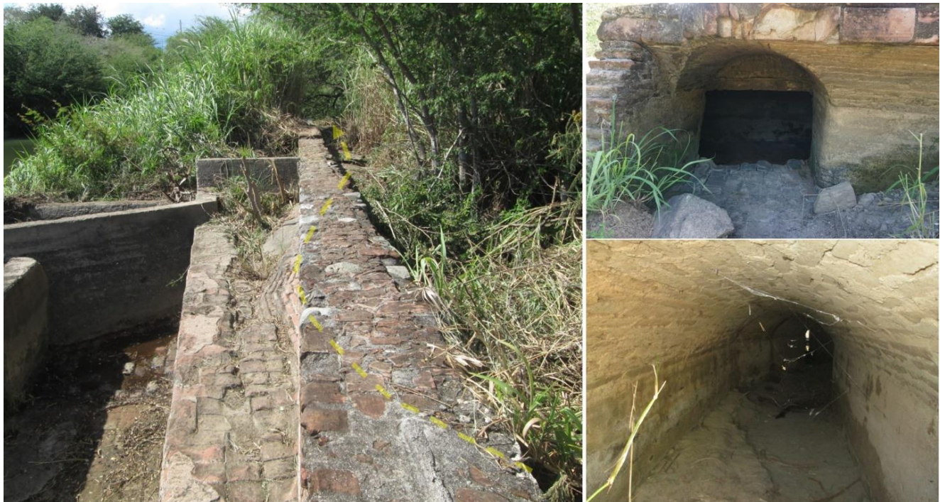
Views of the torrential waters channel. Left; General view of the channels route, marked by the yellow dotted line. Right top; entrance into the supply channel facing west, and inside view of the torrential waters channel looking south.
