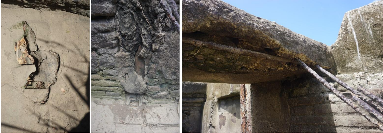
Left and center; remnants of the wood frame of the inner sluice gate of the low waters module. Left; detail of the inner gate of the module, with part of the metal sluice and metal bars that created a garbage trap.
