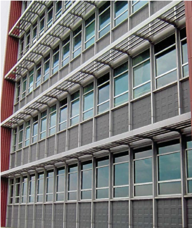
[12] This historic curtain wall features a distinctive variety of panel types which must be repaired or replicated in a restoration project if any are damaged or missing.
