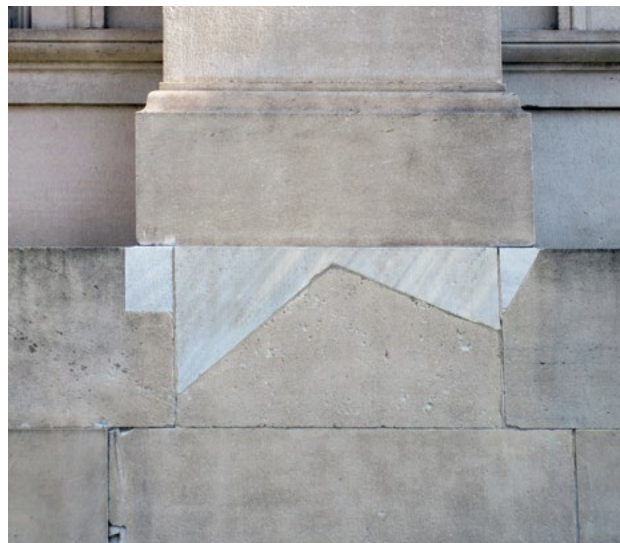
[3] Not Recommended: Although the Dutchman stone repair has been well executed, the replacement stone is not a good color match.
