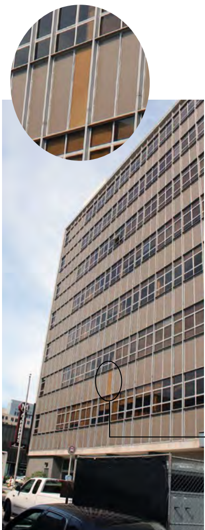
[16] Plywood provides temporary protection for an opening where a damaged spandrel panel was removed until a matching replacement panel can be installed.
