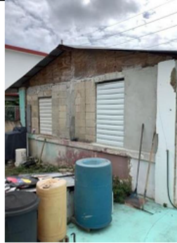
Photo #: 3 Date: August 8, 2023 Description (include direction): Back of Structure, photo direction northeast.
