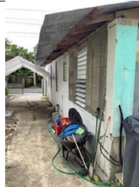
Photo #:4 Date: August 8, 2023 Description (include direction): Right side of structure, photo direction southeast.
