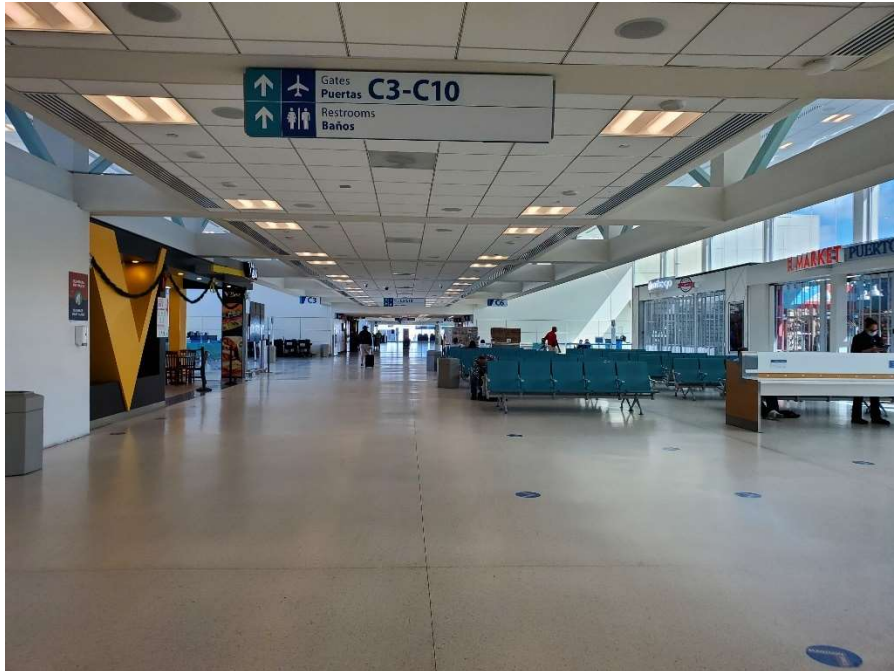
Ilustración 10: "Replace Deteriorating Flooring" Terminal "C"
