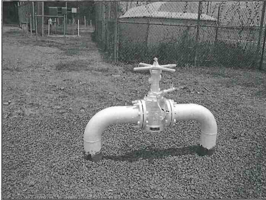
Photograph No. 17 – Test No. 8 Valve Pit 56 DFM Valve No.TFD-128
