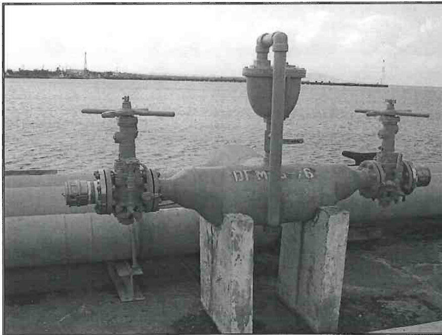
Photograph No. 4 – Test No. 1 DFM-S Valves FP1-100 and FP1-101
