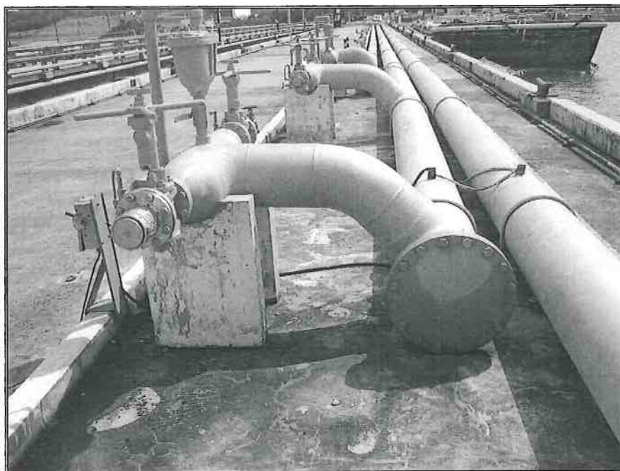
Photograph No. 6 – Test No. 1 DFM Blind Flange Gasket Leak
