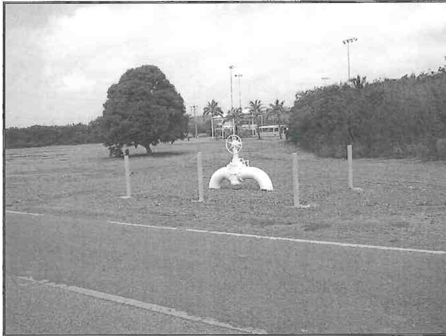
Photograph No. 29 – Test No. 12 Valve Pit No. 8 DFM Valve No.TFD-144
