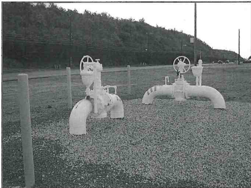
Photograph No. 16 –Pit 24 JP-5 Valve No.TFJ-213 and DFM Valve No.TFD-154
