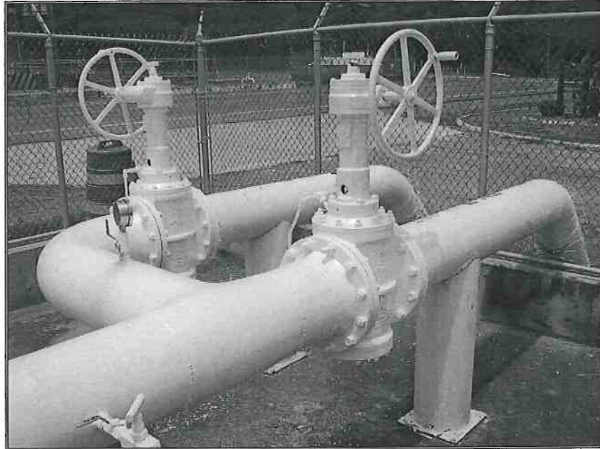
Photograph No. 39 – Test No. 8-Secondary PH 466 Valve No. PH-466-108 and PH-466-109
