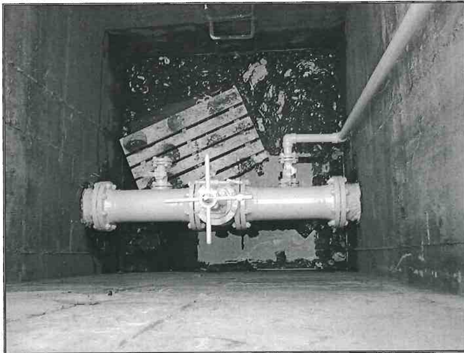
Photograph No. 42 – Valve Pit No.3 Valve No.TFJ-212
