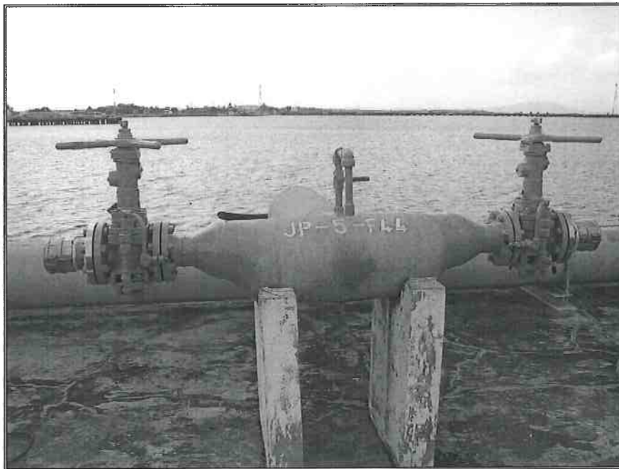
Photograph No. 8 – Test No. 2 JP-5 Valves FP1-110 and FP1-111
