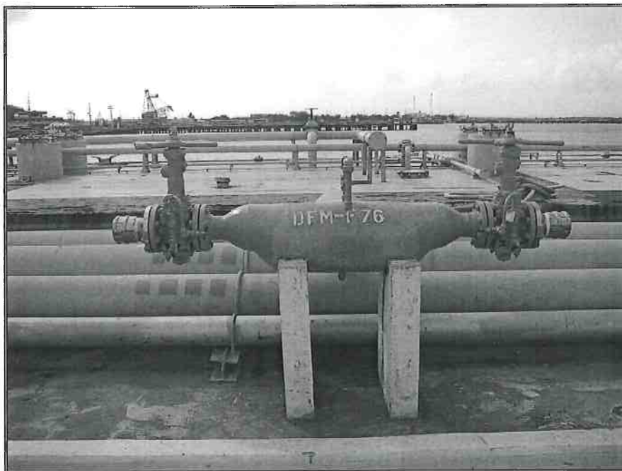
Photograph No. 2 – Test No. 1 DFM Valves FP1-102 and FP1-103
