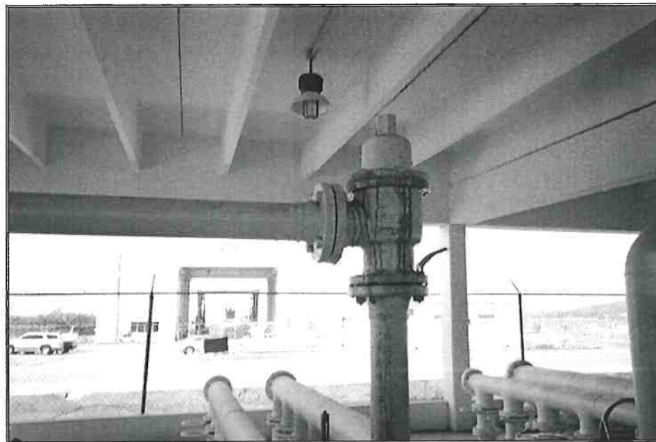
Photograph No. 30 – Test No. 12 Pump Pressure Relief Gasket Leak
