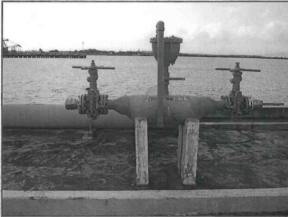
Photo 5A – Pier 1 4-inch Barge Riser with 2-inch Air Eliminator
