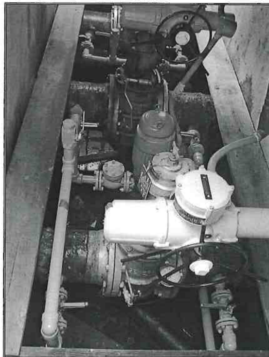
Photo 3C – VP 27 Stripper Piping
