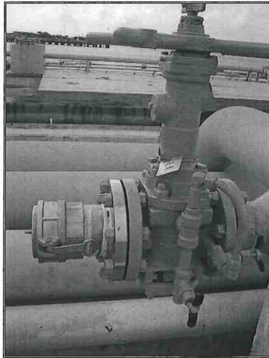
Photo 5C – Pier 1 Barge Riser with 4-inch Camlock Fitting
