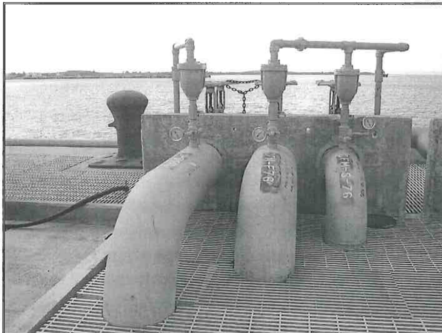
Photo 2A – Pier 1A Air Eliminators
