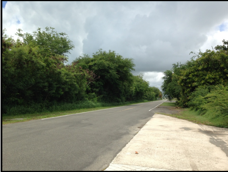
View south along NSRR access road. Poor maintenance observed in picture.
